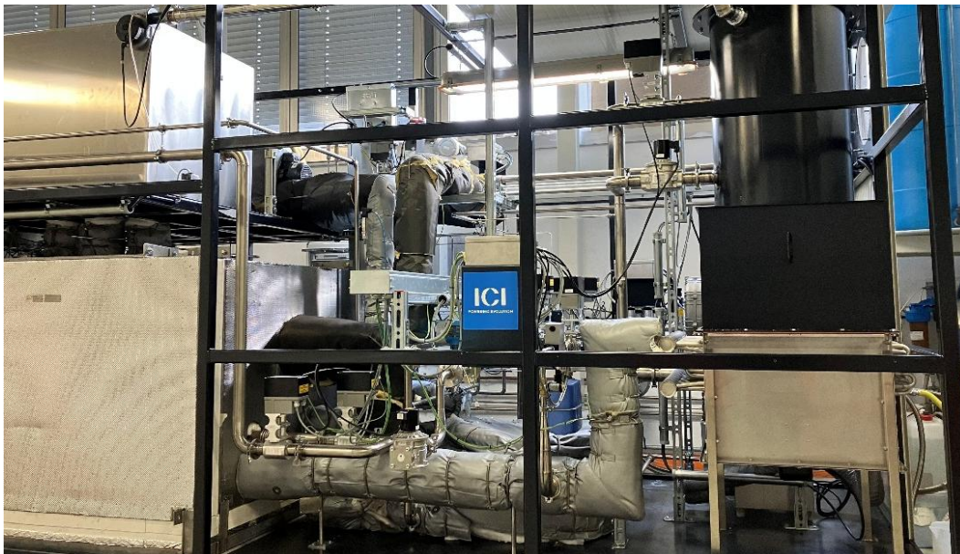
Figure 1 – SO-FREE prototype system integrated at ICI facilities.
